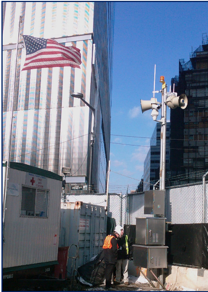
ATI Systems Installation at the World Trade Center
